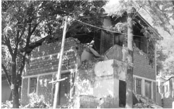
Figure 7.1 : A Damaged Building Due to an Earthquake
